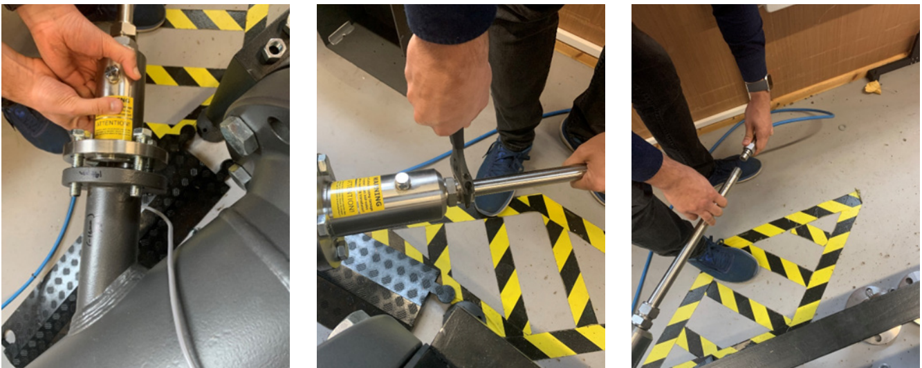
Figure 17. Refitting the transducers into the line
